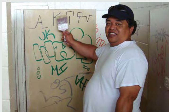
Top photo (from left): Aina Kamaka and John Branco work to repaint the restroom walls at Kāneohe District Park. Bottom photo: Lincoln Hose paints over a door covered in graffiti.
